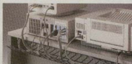
Wire mesh cable management neatly routes cables along the back of tables, allowing equipment connections at convenient points.
