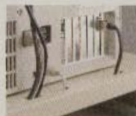
Cables are neatly channeled to the rear.
